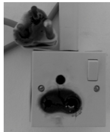
Figure 2: Burned wall socket
